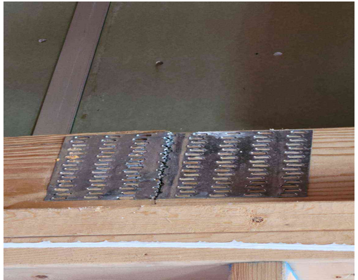
Broken gusset plate on left wall in master bedroom.
