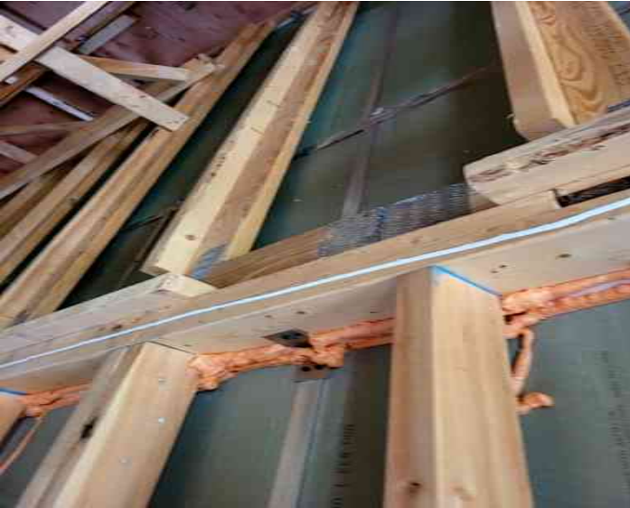
Broken gusset plate on left wall in master bedroom.
