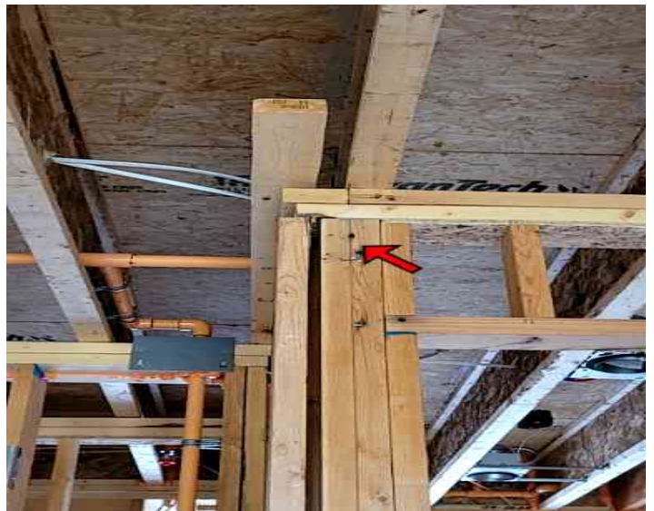
Doorway framing in kitchen not flush and should be repaired.
