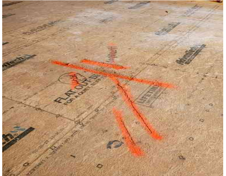
Scuffed subfloor in master bedroom and should be repaired.
