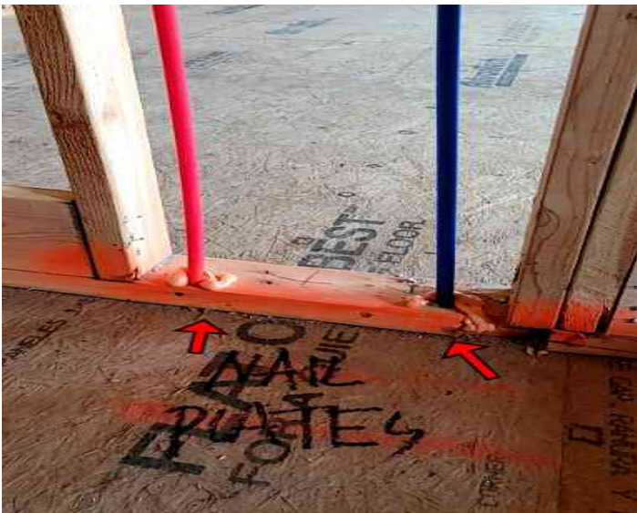
Missing nail plates were noted in master bathroom tub/shower and should be installed.
