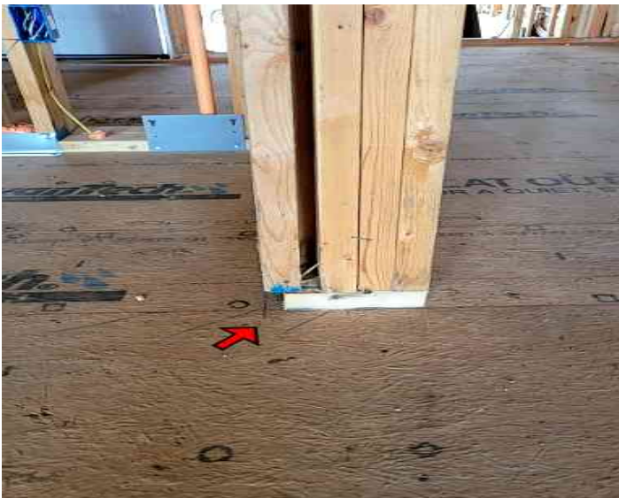
Doorway framing in kitchen not flush and should be repaired.
