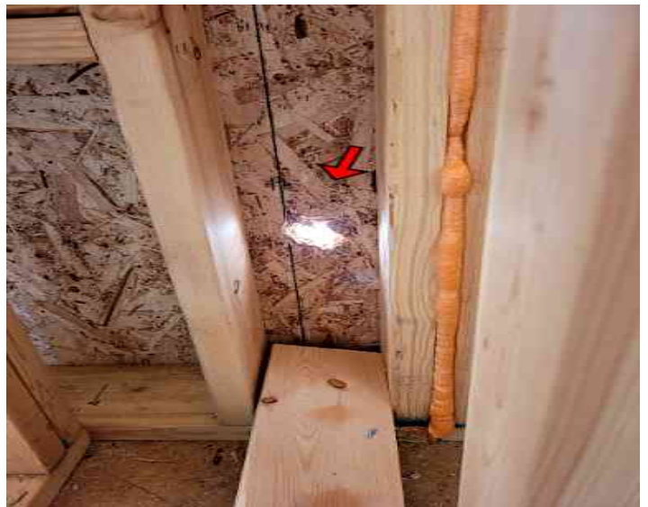
Gap in exterior wall noted in master bathroom closet and should be sealed prior to drywall and insulation installation.
