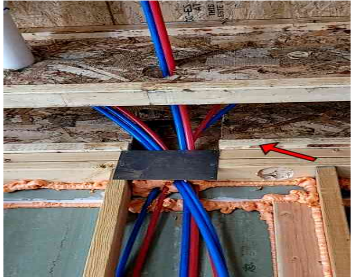
Right wall kitchen compromised truss/joint and should be evaluated and repaired.
