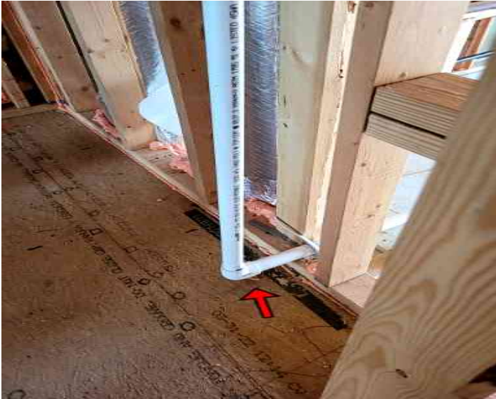
Drain pipe outside of wall cavity in half bath was noted and should be repaired.
