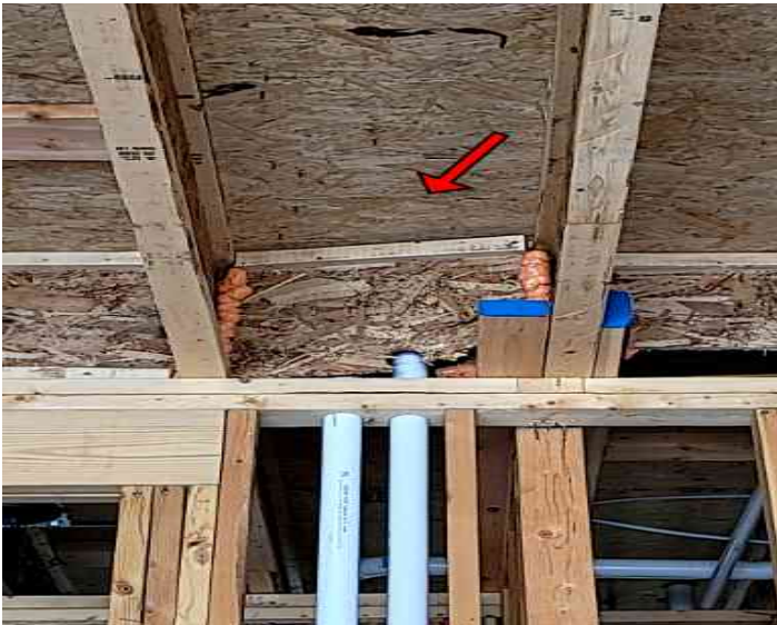
Poorly fitted and sealed blocking was noted on a rear wall and should be repaired.
