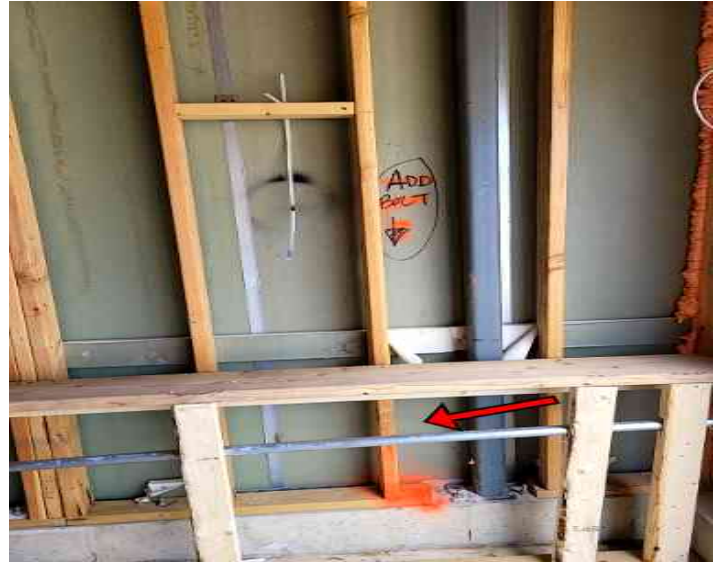
Twisted stud noted on right wall and should be repaired.
