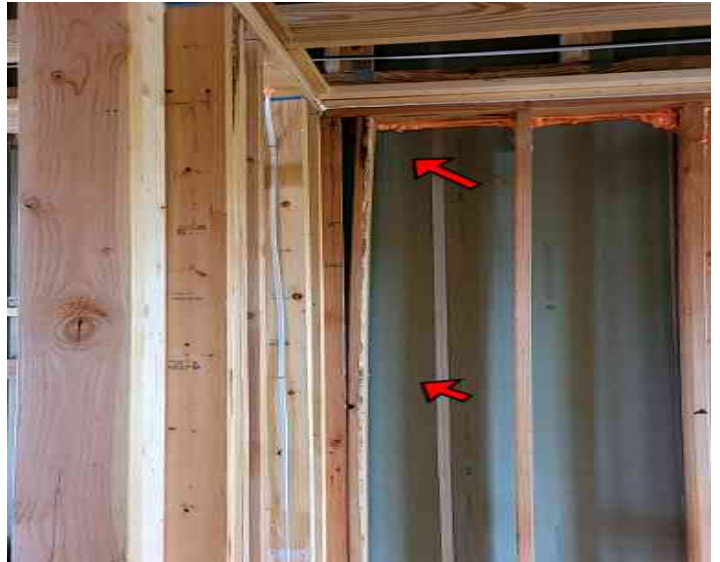
Poorly framed stud on 2nd floor left wall in stairwell and should be repaired.
