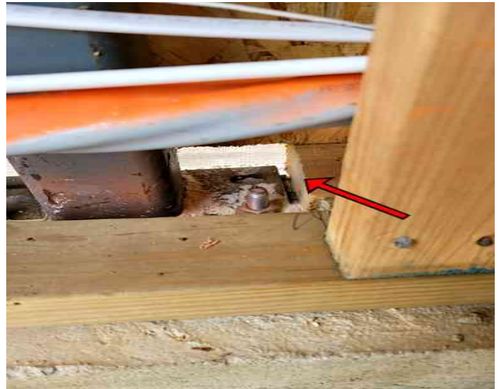
Gap/daylight was noted on left wall and should be repaired.
