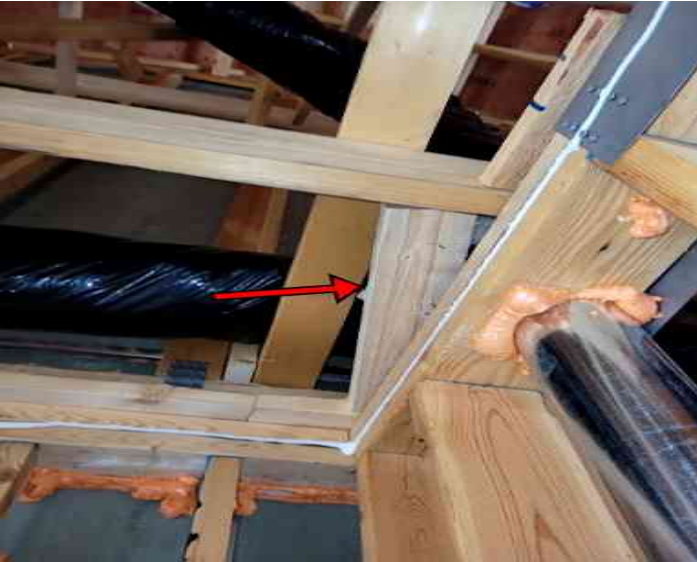
Poorly installed nailer was noted in 2nd floor middle right room and should be repaired.
