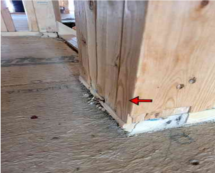
Exposed nail noted right of basement stairs and should be repaired.
