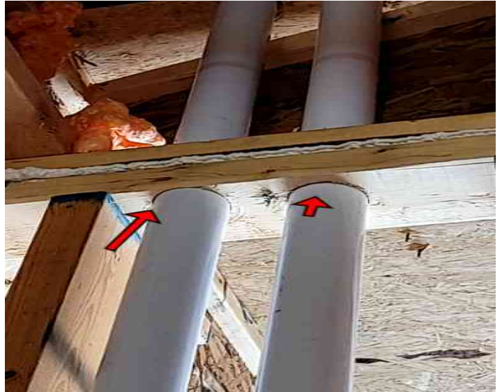
Missing nail plates left of garage door were noted and should be installed.
