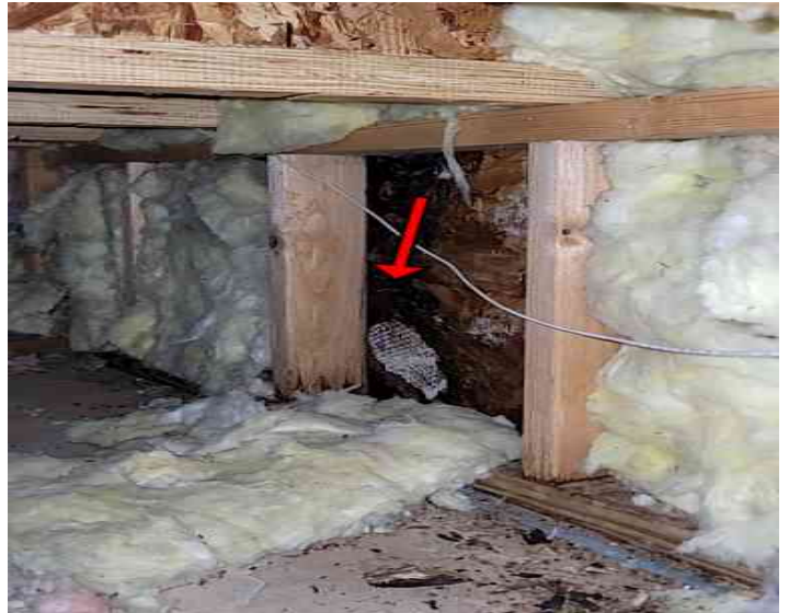
Damaged sheathing and rot noted also exposed lath
