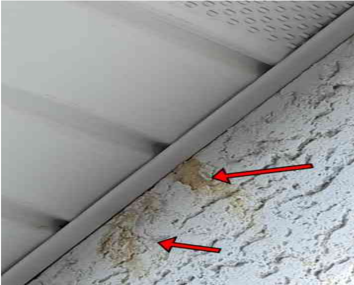
Stains at front soffit indicate leakage
