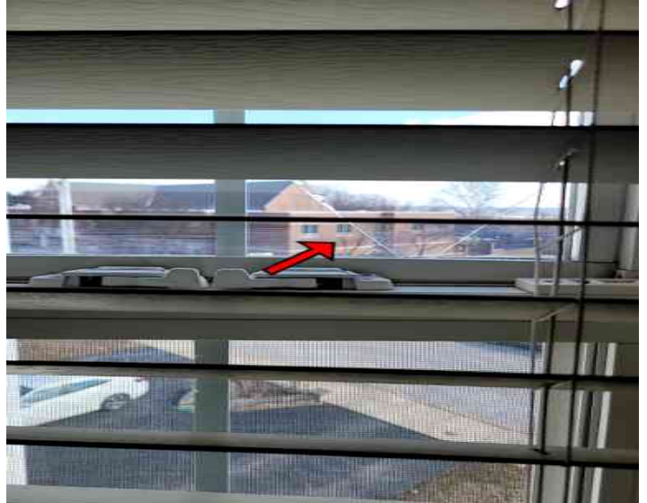
Master bedroom left window cracked
