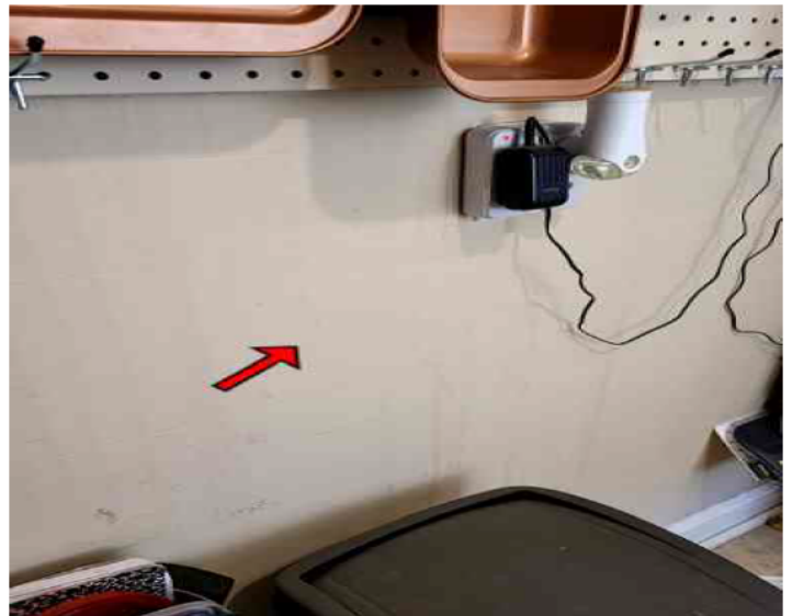
Apartment 1 kitchen water stains.
