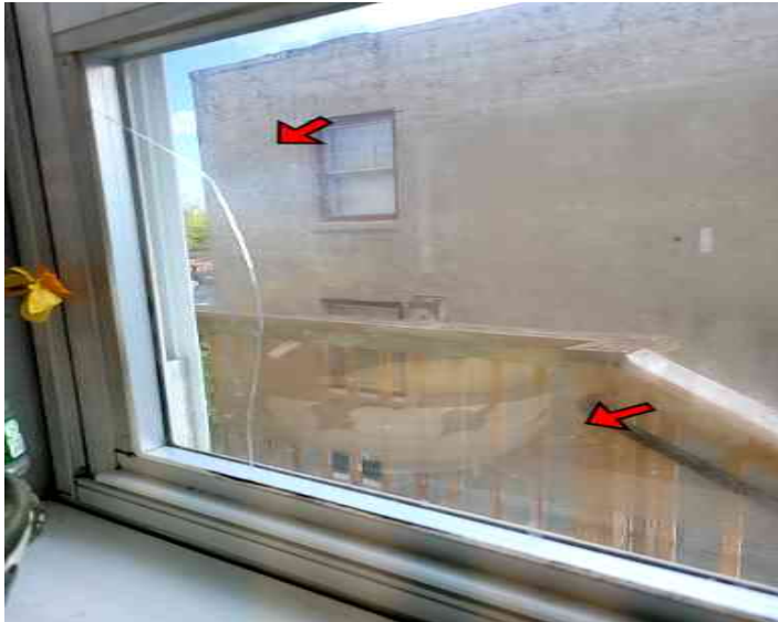
Apartment 1 kitchen. Broken glass and condensation.
