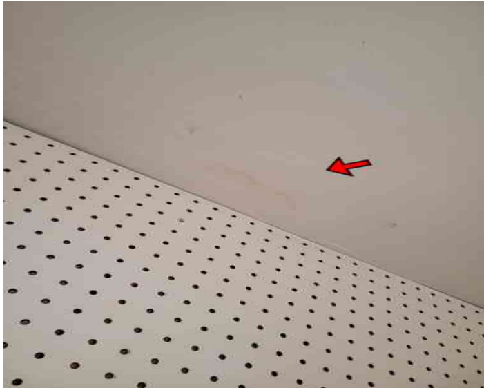
Apartment 1 stain was noted but was dry at time of inspection.
