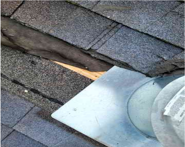
Exposed sheathing noted.
