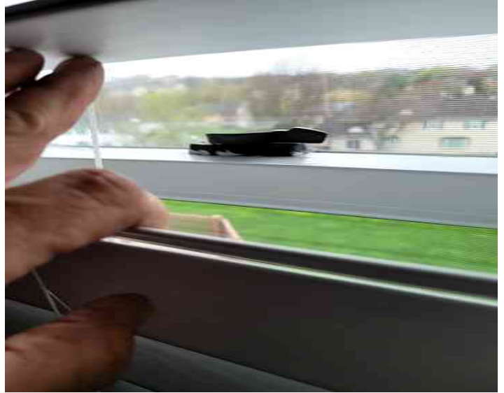
Rear right bedroom window would not lock
