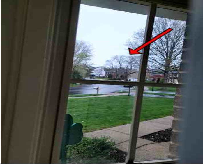
Damaged balances in bay window
