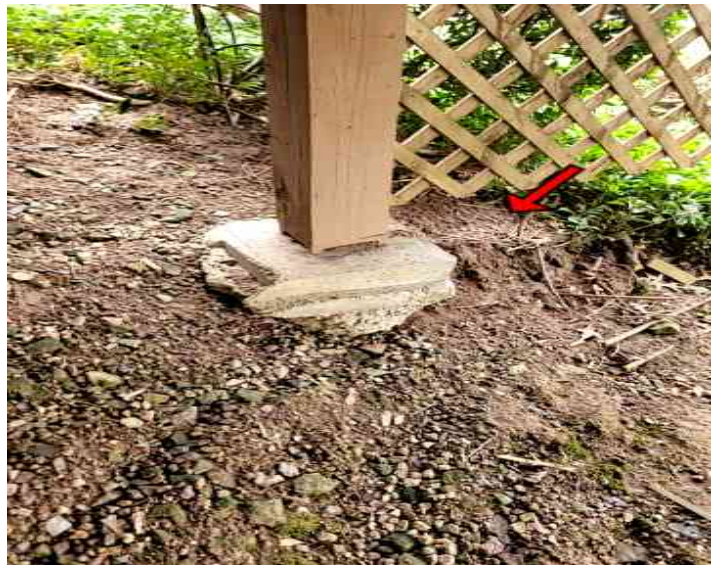
Some erosion at footing
