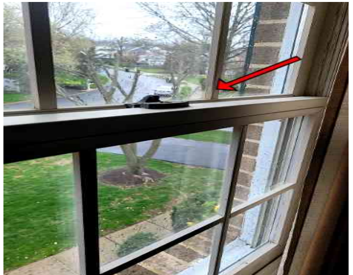
Missing Hardware master bedroom
